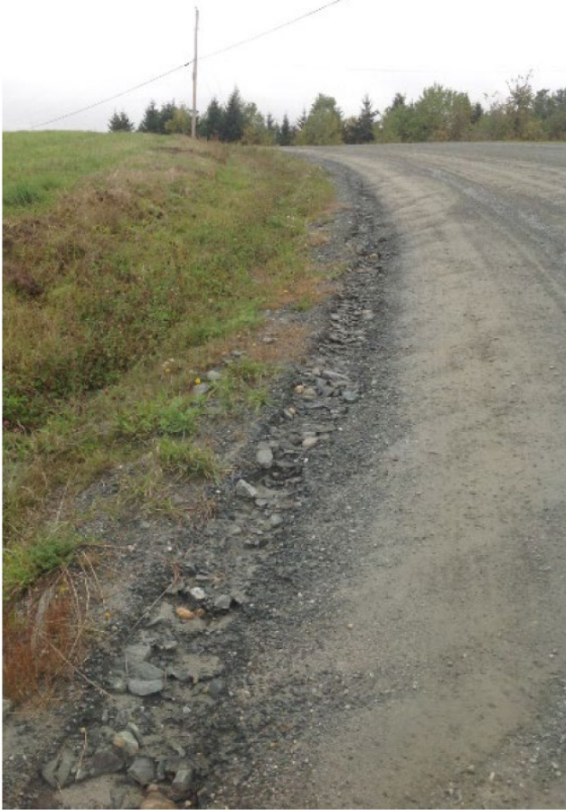
Figure 66: Segment 121209- heavy erosion on north side of road
