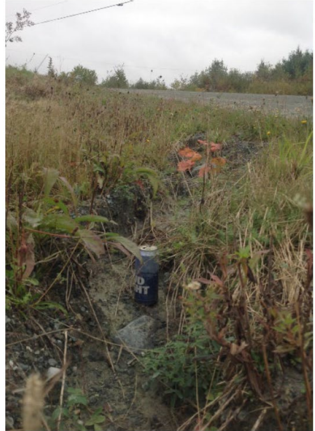
Figure 67: Segment 121209- scouring occurring
