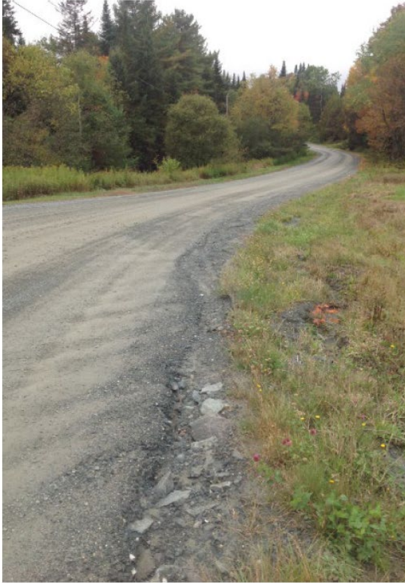
Figure 66: Segment 121209- turnout full of sediment
